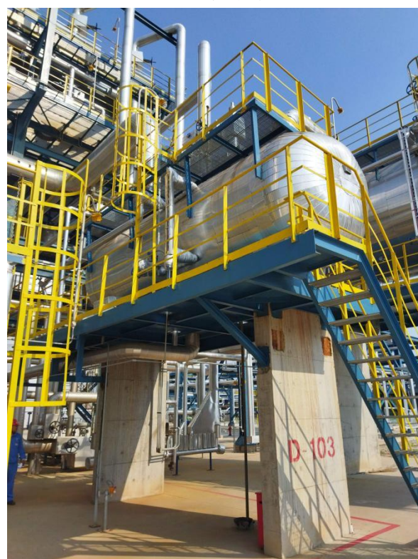
汽提塔顶回流罐
